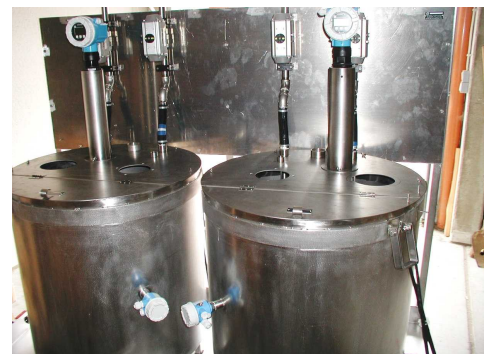
400 l store tanks for production, incl. level control
